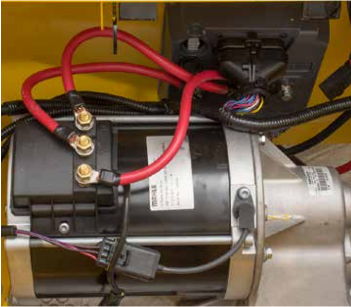
Figure 15: The motor connected to the Sevcon motor controller.
