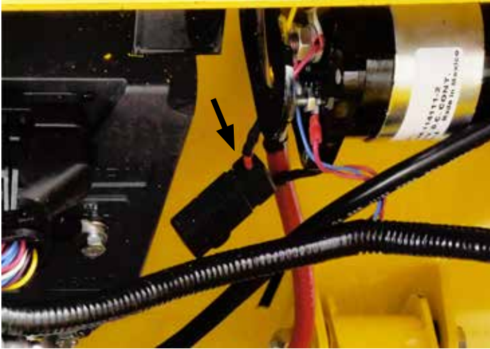
Figure 9 The fuse (indicated by the arrow) should be removed before performing any maintenance or repair work on the electrical system.
